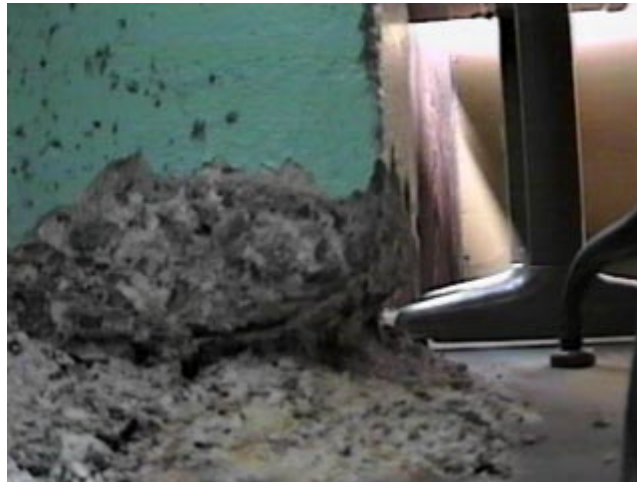
PHOTOGRAPH NO. 1 - Crumbling concrete column in basement of Garfield Elementary.
