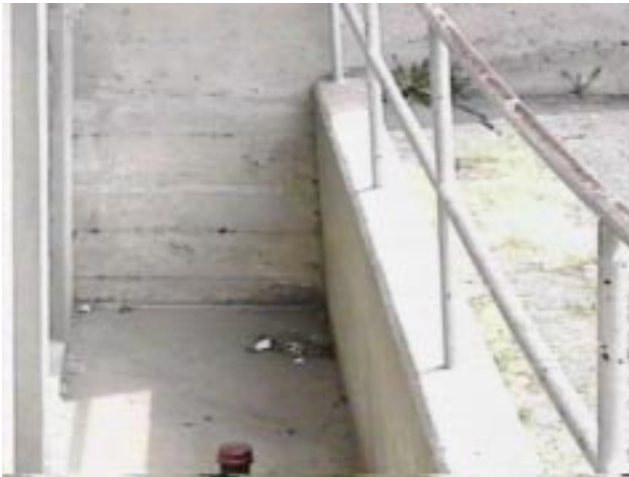
PHOTOGRAPH NO. 3 Window well retaining wall overturning from weight of soil.
