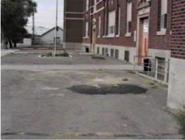
PHOTOGRAPH NO. 4 Water ponds at many areas around base of building and window wells due to flat ground surface.
