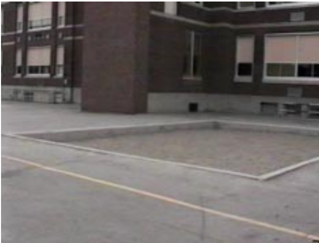
PHOTOGRAPH NO. 5 Wind blows sand from sandbox to window wells.
