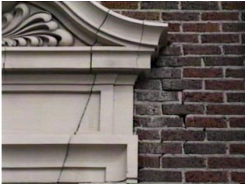
The exterior of Garfield School is in need of maintenance. This photo shows brick that needs repointing.
